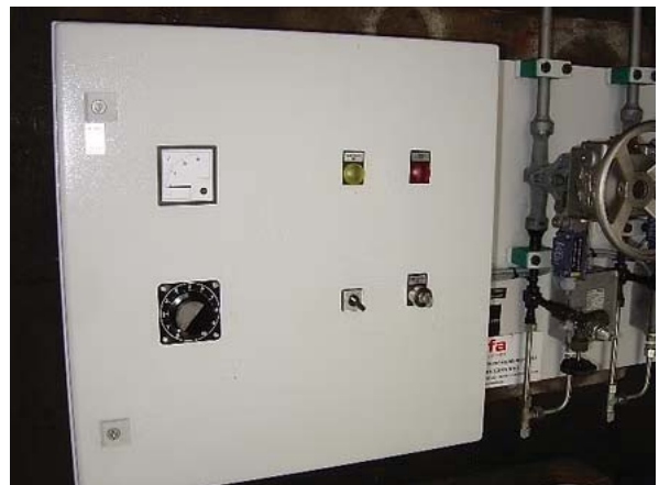
Electrical testing device
